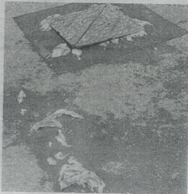
Excrement appeared to have been pushed from under a manhole cover
